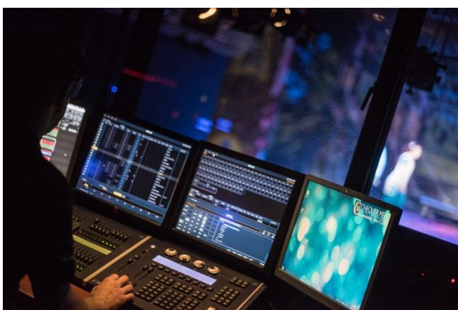
View from the Control Room
